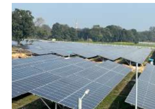
MONDELEZ INTERNATIONAL Induri MAHARASHTRA 2.7 MWp
