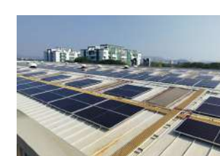
JUPITER WAGONS Metal Shed Grid Connected MAHARASHTRA 0.9 MWp
