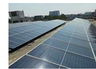
RAGHAV LIFESTYLE RCC Rooftop Behind the Meter HARYANA 1.0 MWp
