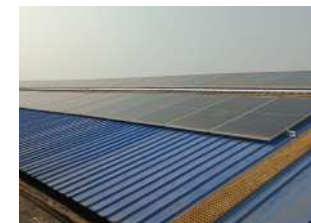
MONDELEZ INTERNATIONAL Captive Open Access MADHYA PRADESH 2.6 MWp
