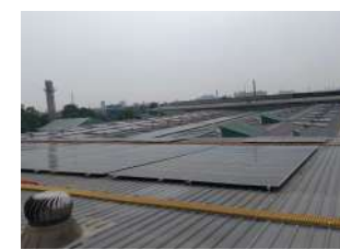
JINDAL ALUMINIUM Metal Shed Rooftop Behind the Meter RAJASTHAN 3.0 MWp
