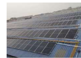
BIRLA JUTE MILL Metal Shed Rooftop Behind the Meter WEST BENGAL 2.1 MWp
